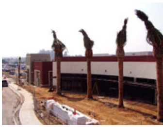
Placing these palms required street closure, cranes and more than two days of meticulous labor.
